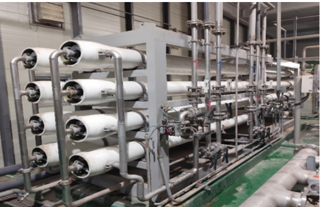
CWRO (Concentrated Water Reverse Osmosis)
